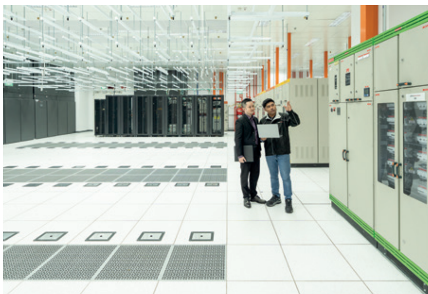
Keppel leverages its operational expertise in data centres and power to future-proof data centre infrastructure by deploying artificial intelligence and machine learning, as well as incorporating sustainable design and energy-efficiency solutions.
