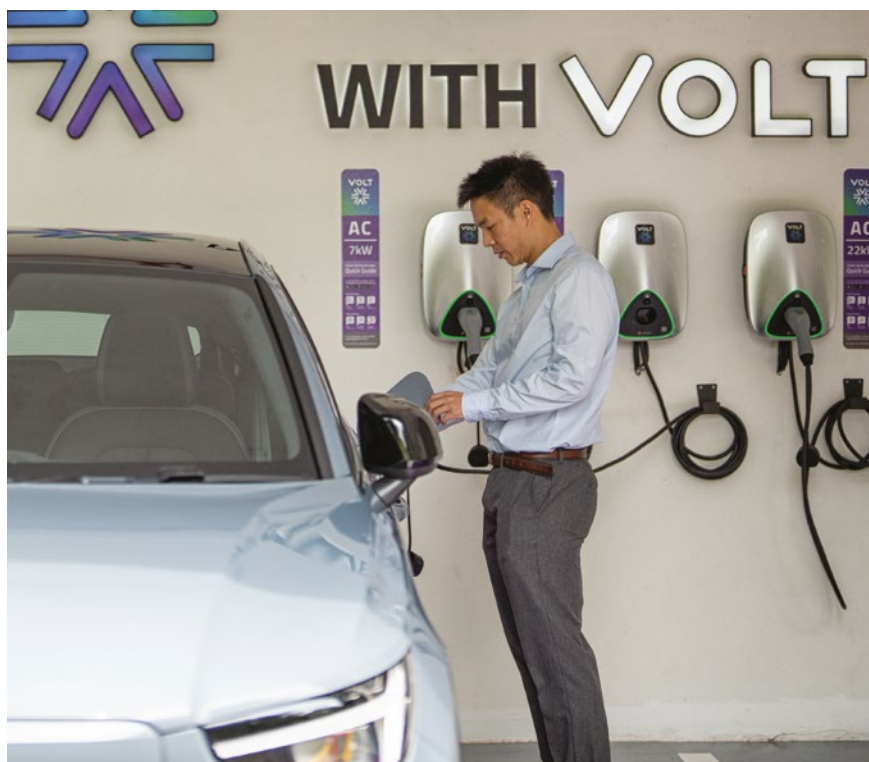
Keppel continues to expand its customer base for EaaS offerings, such as district cooling, solar panels and EV chargers.
