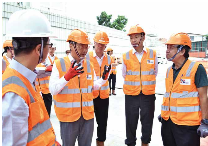
Keppel's Board Safety Committee regularly conducts site visits to the Group's projects such as The Garden Residences in Singapore.
