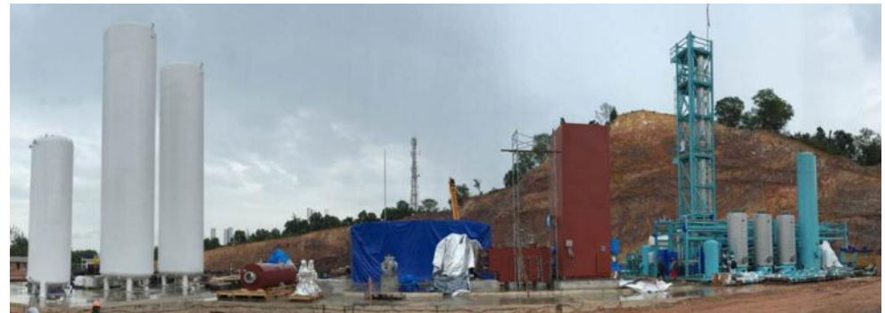
The land-based PreNEx LNG plant for PT NAT Gas has a liquefaction capacity of 50 tons/day.
