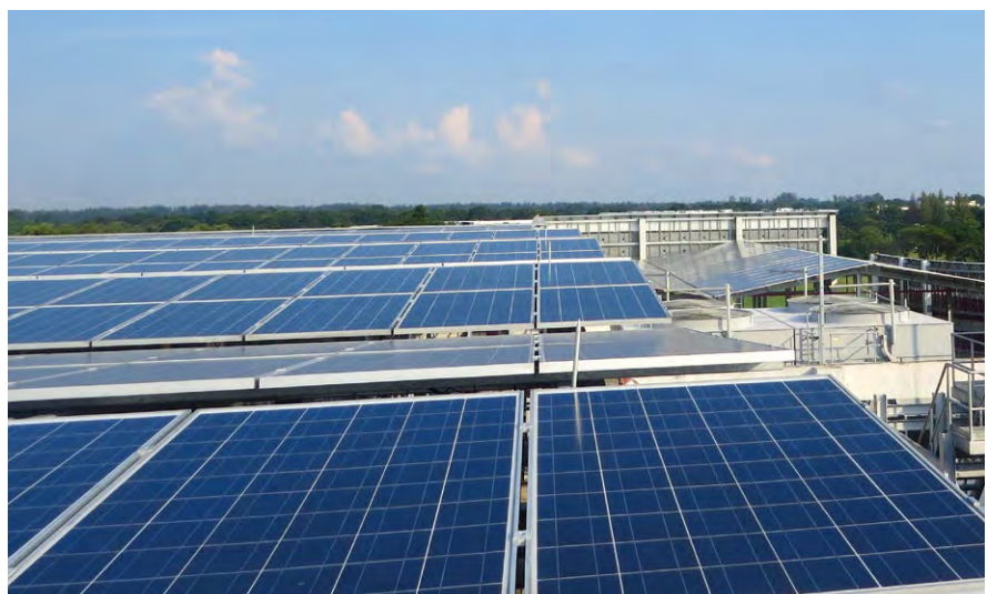
Keppel Land's corporate office at Bugis Junction Towers is fully powered by solar energy from Keppel Electric.
