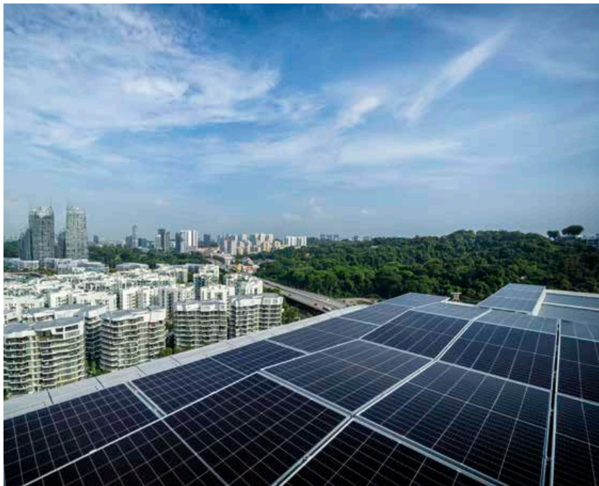
Installation of the photovoltaic panels at Keppel Bay Tower was completed in March 2021, generating an energy yield of about 100,000 kWh per annum.
