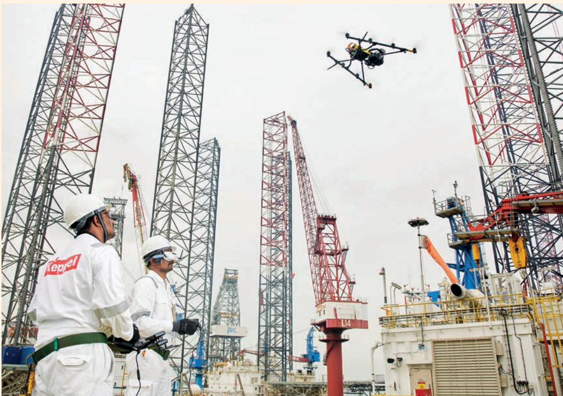
Utilising drone technology, Keppel is able to safely and efficiently inspect, analyse and provide repair support in high-risk and difficult to access areas.
