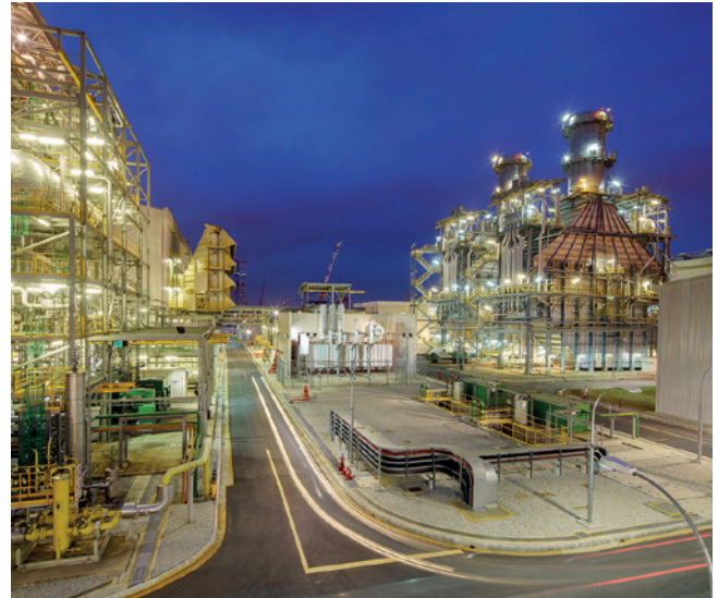
The upgrade of the Keppel Merlimau Cogen is estimated to contribute up to 8,000 tCO 2 e of avoided emissions in 2023, compared to the emissions prior to the upgrade.
